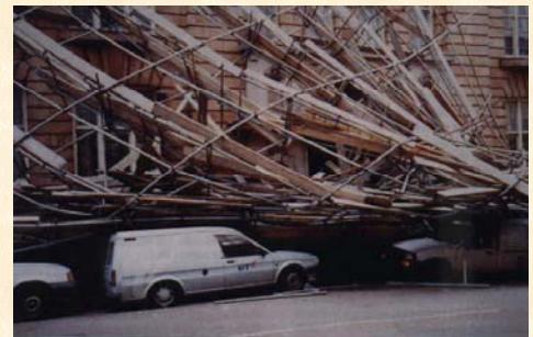
The collapsed structure
