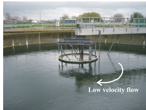
Figure 2.8. Rotary Sludge Separation.
