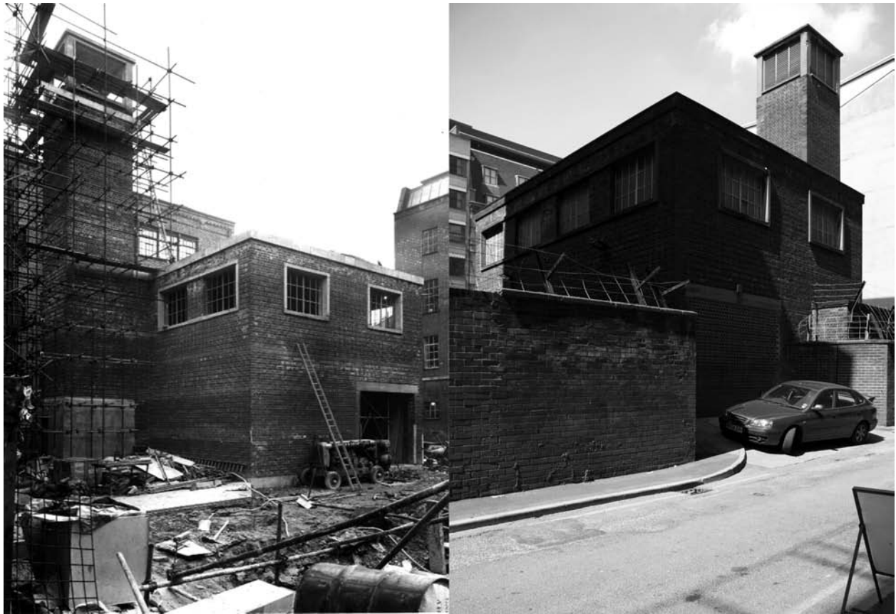
Figure 3. [image left] Original photograph documenting the construction of the service building at 56 George Street, Manchester, dated November 1960. Photograph taken inside the compound. The distinctive exhaust tower is nearly complete. (Source: Photograph by tunnel engineer Patrick Gough. Courtesy of George Coney.) [image right] A contemporary view of the utilitarian same building at the top of the main equipment lift shaft down to the GUTE . The compound now features significant physical perimeter security. Photograph taken from Back George Street (Source: Richard Brook).
