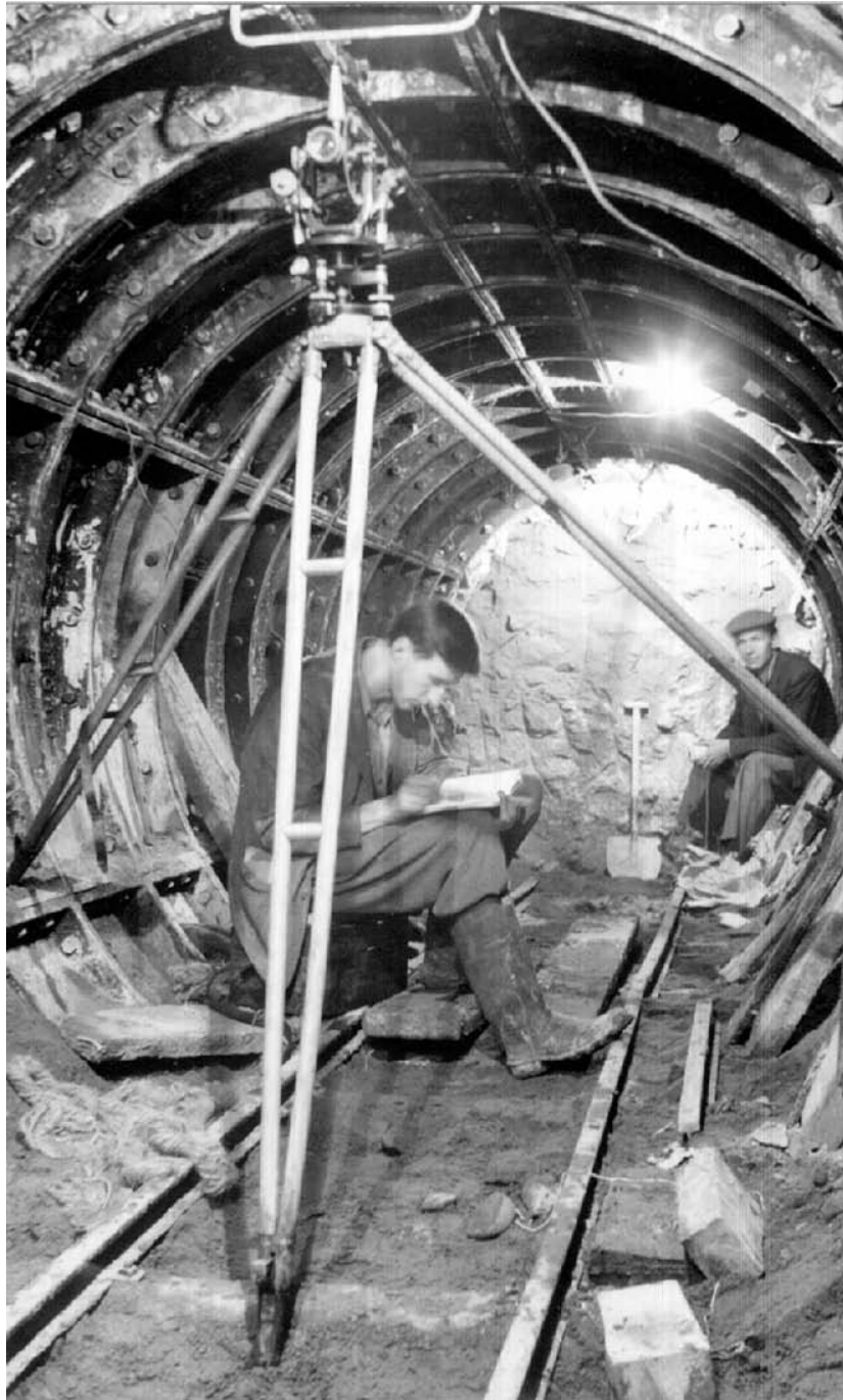
Figure 7. Original photography documenting the construction of the GUTE , dated June 1955. Survey work in progress on one of the smaller cable tunnels. (Source: Photograph by tunnel engineer Patrick Gough. Courtesy of George Coney.)
