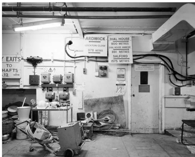
Figure 4. A July 1988 photograph of signage in the cable tunnel crossover indicating the scale of the distances to various exit shaft for GUTE. Ardwick 978 metres to the left and Dial House 900 metres, with Salford 1575 metres to the right. (Source: Tony Perry, English Heritage, ref. AA98/02434).
