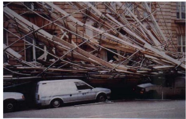
b) The collapsed structure
