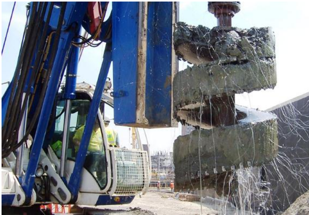
Figure 1.2 A twin flight auger immediately after being extracted from a hole supported by a polymer fluid (Lam et al. , 2010).
